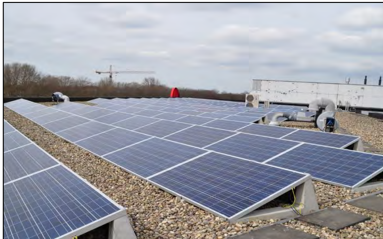
Figure 32 Solar Power Plant at Sirajudeen Nagar
